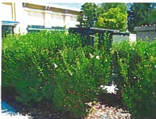
Exterior utility equipment screened with planting
